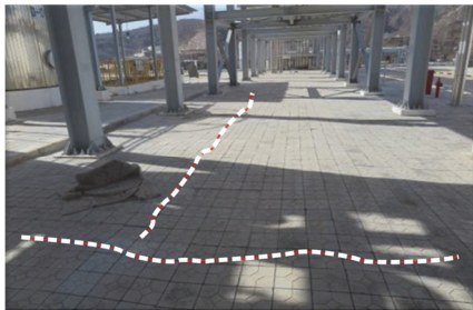
图 2 靖边某天然气厂区湿陷沉降 Fig.2 Subsidence of a natural gas plant in Jingbian
